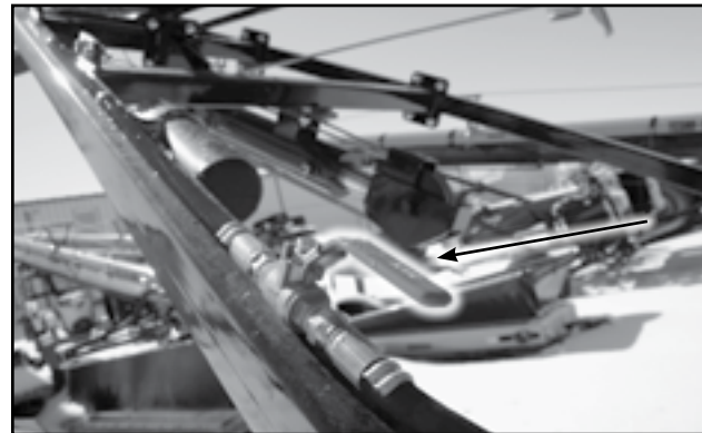
Fig 11 - Hydraulic valve to the lift cylinder
